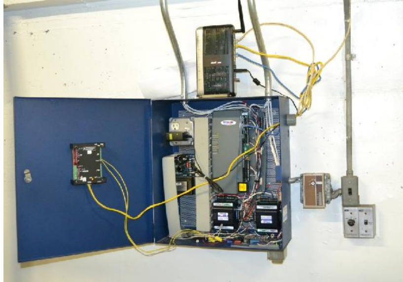
Figure 12. Electronic controls and Internet connections provide for remote monitoring of plant operations.
