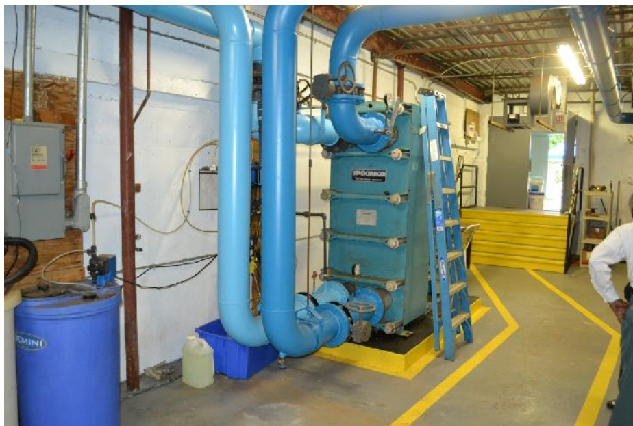
Figure 9. Cold water heat exchanger.
