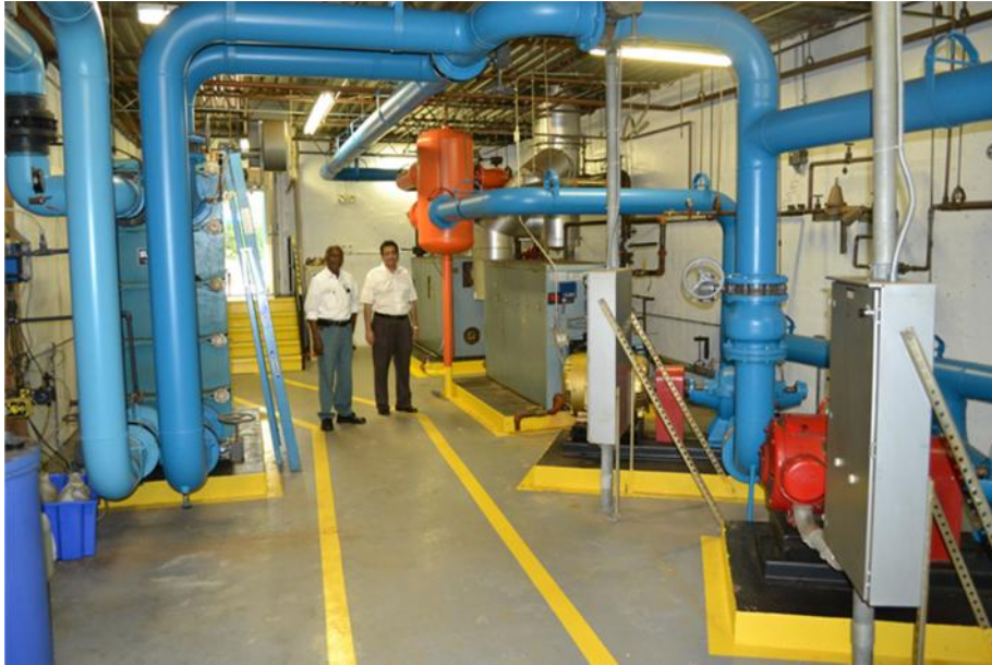
Figure 8. Inside a Plant. Lightest blue pipes are for cold water, darker blue pipes for hot water.
