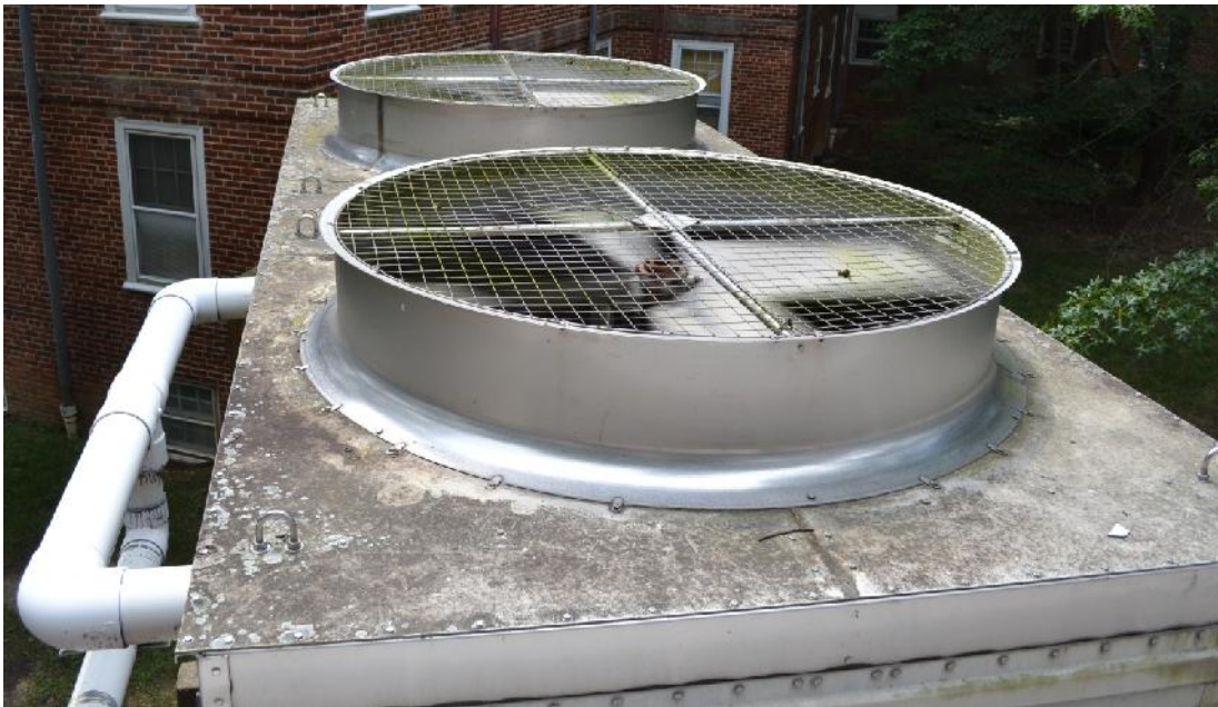
Figure 13. Cooling tower fans.
