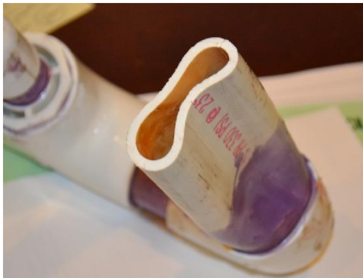
Figure 7. Melted HVAC PVC Pipe
